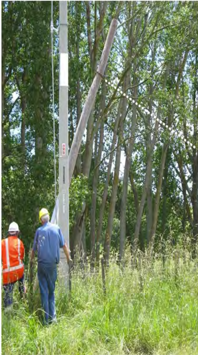
Photo 23: Pole 125668 at failure. Chain highlighted.
