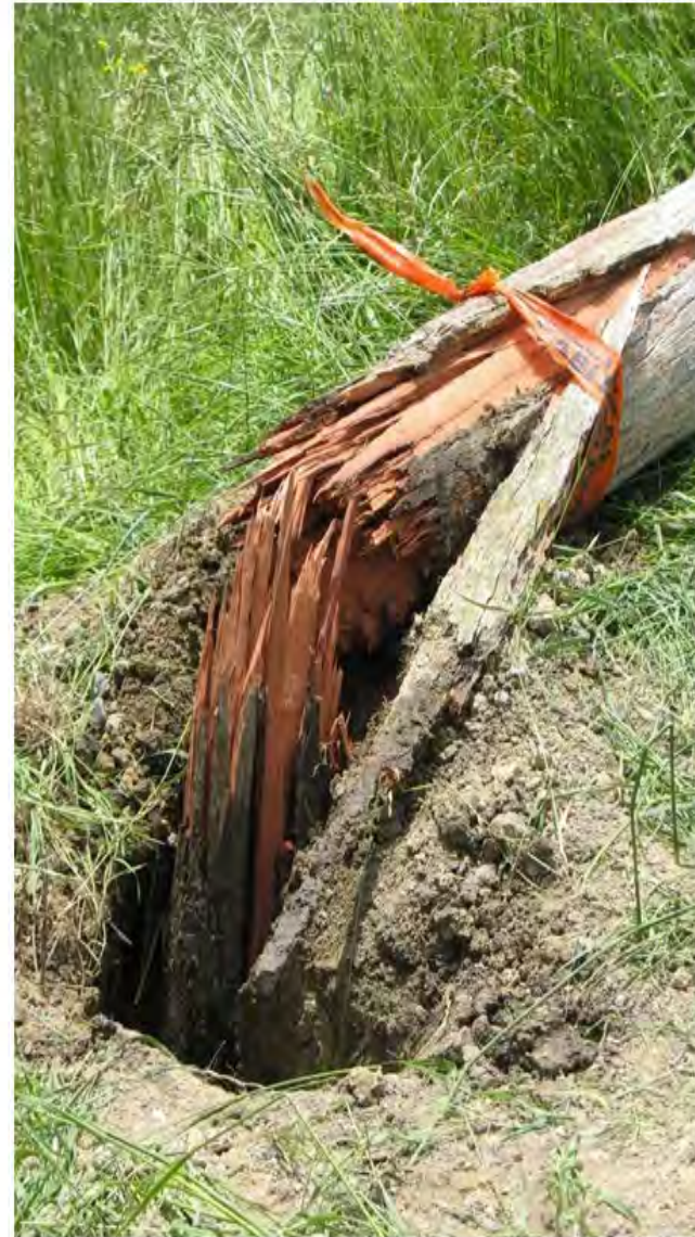
Photo 24: Fracture in base section of Pole 125668.
