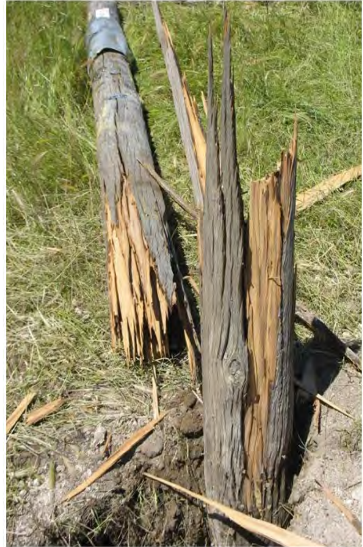
Photo 18: Fracture in base section of Pole 135134.
