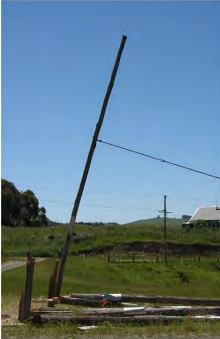
Photo 17: Pole 135134 at failure.
