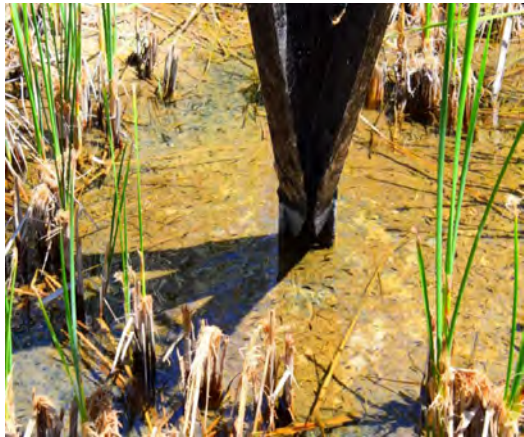
Submerged Pier and Stub Angle
