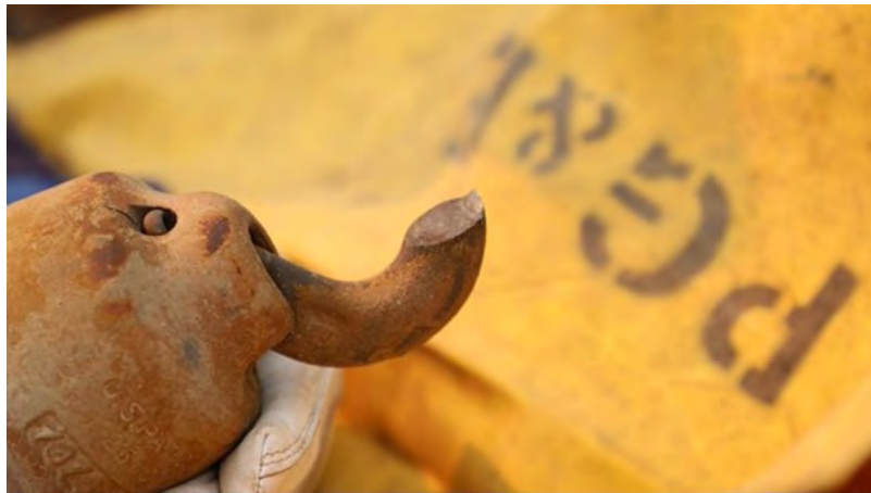
97year hook fractured due to fatigue
