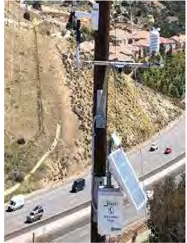
New electric utility equipment
